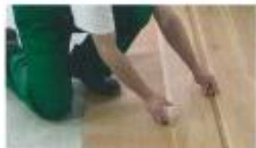
Fig. 3. The view of 3-layer wooden floorboard produced by Barlinek Inwestycje Sp. z o.o. during installation
